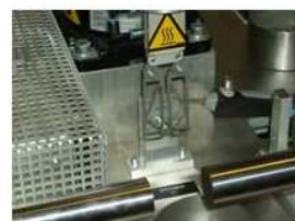
Surface temperature control
